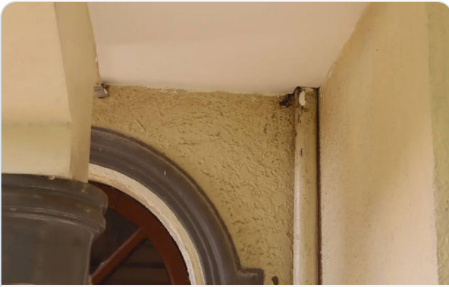
PHOTO 15 · PORCH CEILING CORNER
